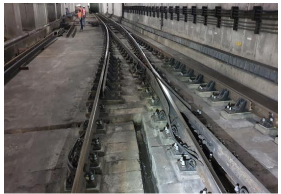
Fig. 3. Renewed Turnout (DTRO)
