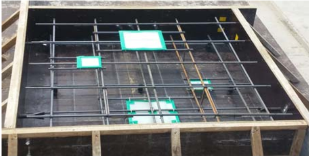
Fig. 1 Installation of reinforcing steel mats and fabricated delamination in a wooden concrete form before casting concrete.
