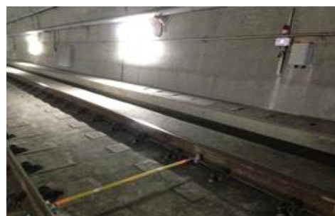
Fig. 1 Installation status of measurement sensor
