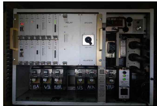
Fig. 6 ATC Onboard Signal Equipment with Developed CFA & Power Supply
