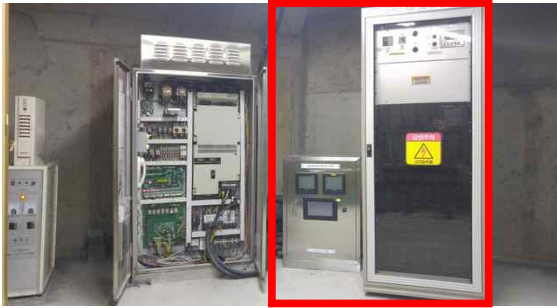
Fig 1 Installation of elevator ESS and energy analysis system
