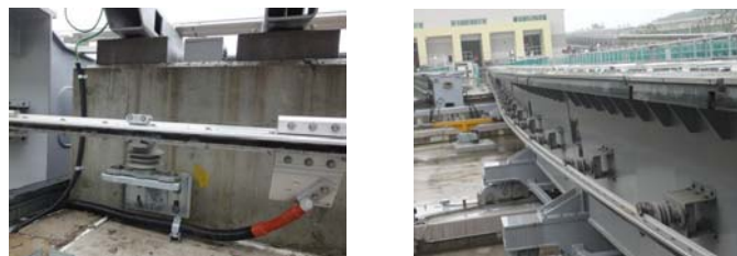
Fig. 1 Insulator installed in Maglev railway line
