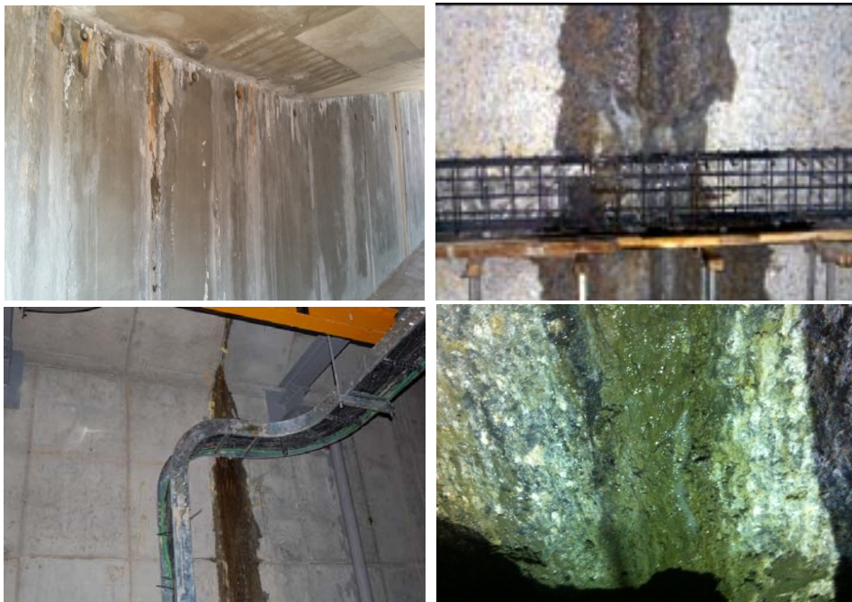
Fig. 1 Example of Leakage for Precast Module Connection Joint
