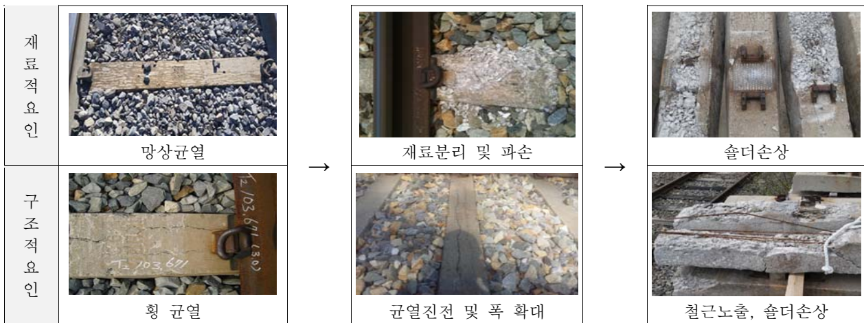
Fig 1. Representation types of damage of PSC sleeper
