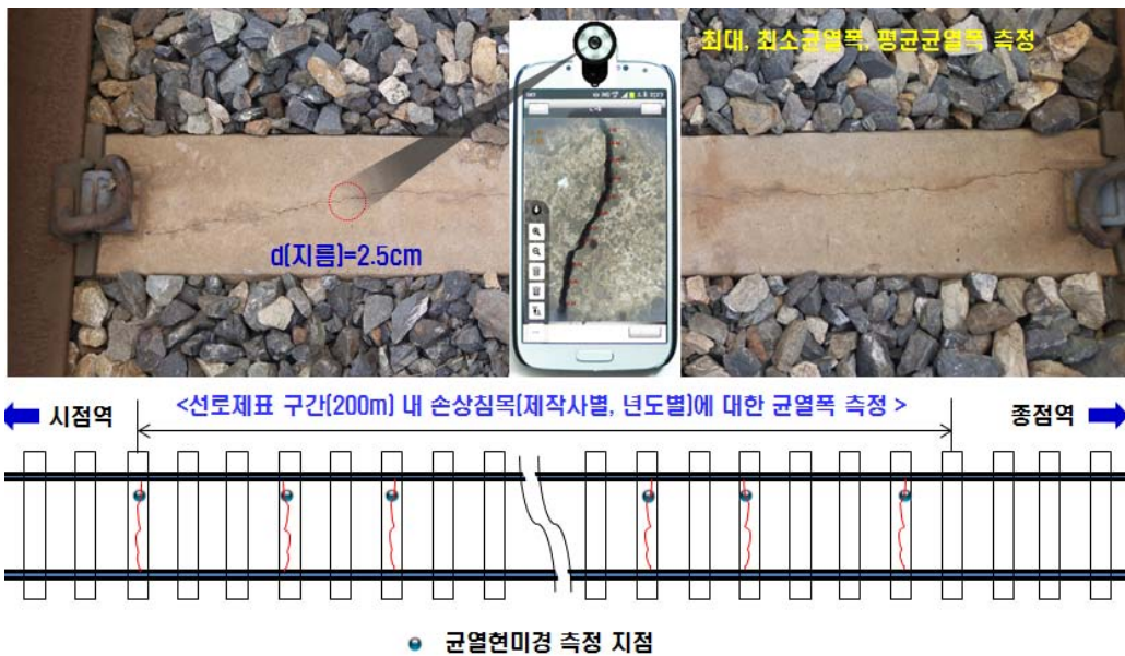
Fig 2. Crack width measurement of PSC sleeper
