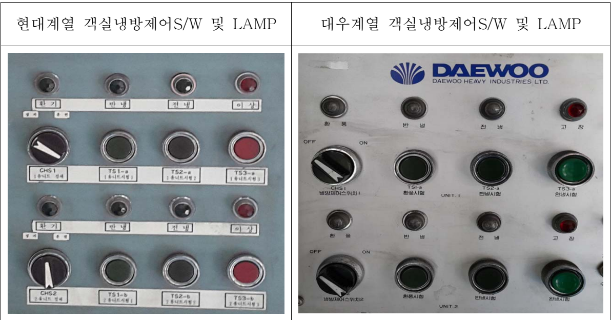
Fig.1 Heating and cooling circuit Panel in the cabin
