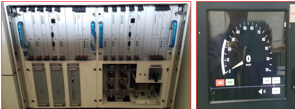
Fig.4 ATC device and ADU YARD display
