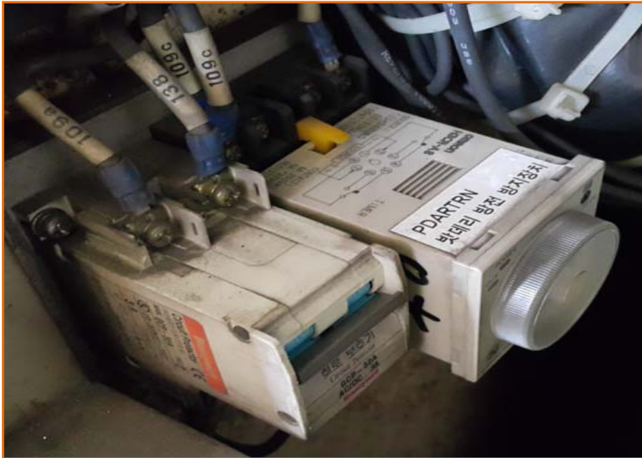
Fig.4 discharge protection circuit in the box of pane
