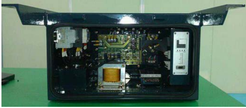
Fig2. Compressor Motor Starting Box - Maglev
