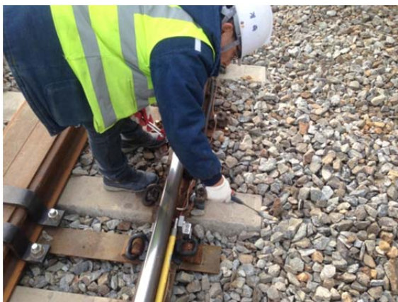
Fig. 9 Rail-mounted displacement sensor installation
