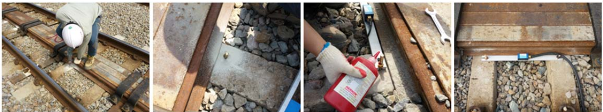
Fig. 2 Installation example of typical rail displacement monitoring system
