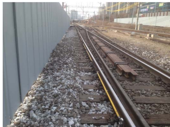
Fig. 10 Site view after sensors installation
