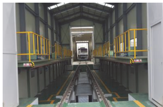
Fig. 6 The interior of the lower washing equipment
