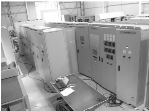
Fig. 1 Active Harmonic Filter
