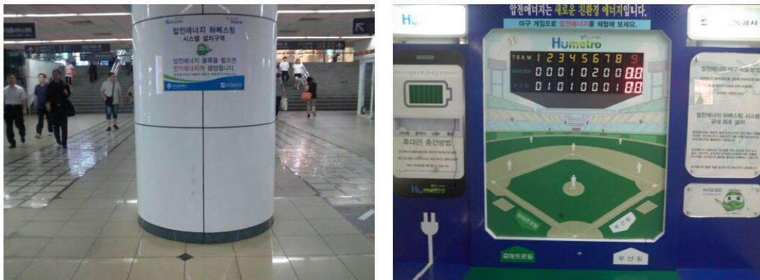
Fig. 2 piezoelectric power generation system, Seomyeon Station in Pusan
