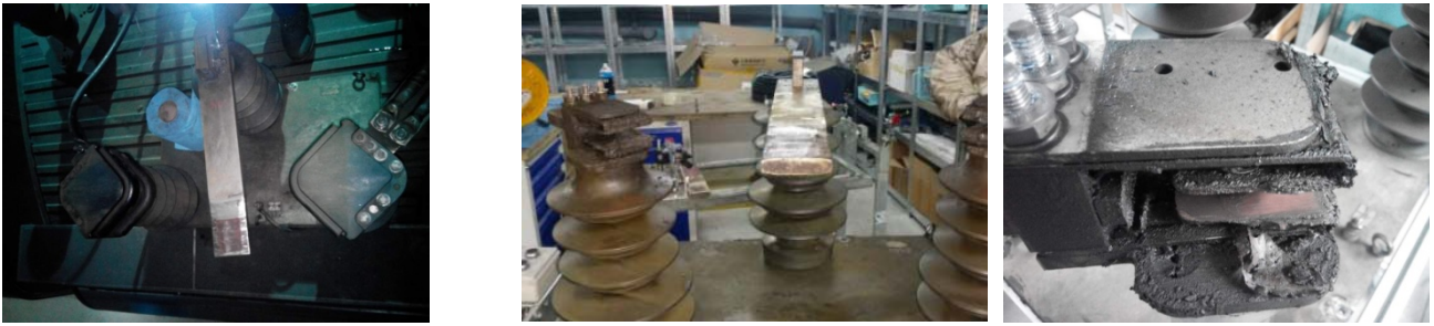
Fig. 2 Damaged ADCG (Ex. Ukraine EMU)
