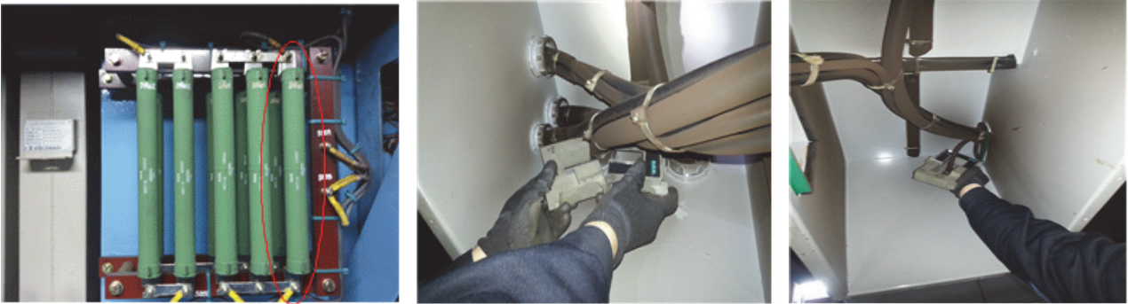
(a) Measuring point of voltage
